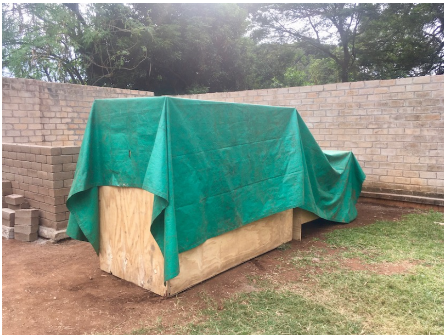
Figure 3: Delivered essence extraction equipment at MMCT offices.
